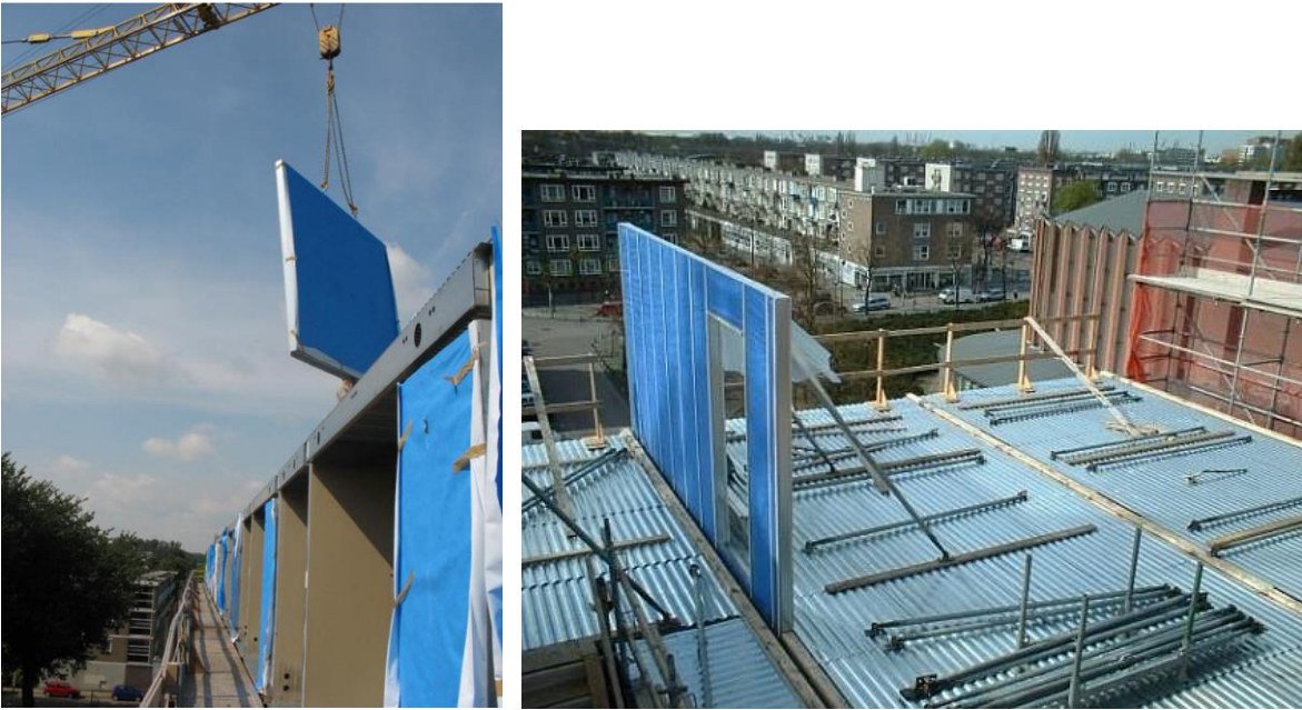
Figure 34: Rooftop retrofitting example, only 'dry' building techniques are used; highly prefabricated Project Lage landen (publicatie Bouwen met Staal)
